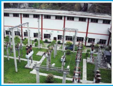
Outside View of Hunan Daxing Powerstation
