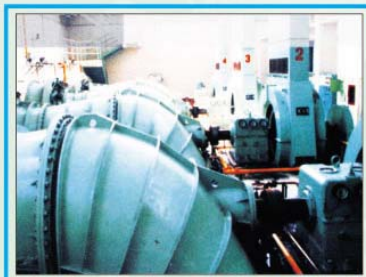
Hunan Xiangshui Powerstation with 4x1.25MW Tubler Turbine Units
