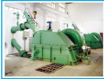
Hunan Daxing Powerstation 3x2.5MW Pelton Turbine Units with Double Nozzles
