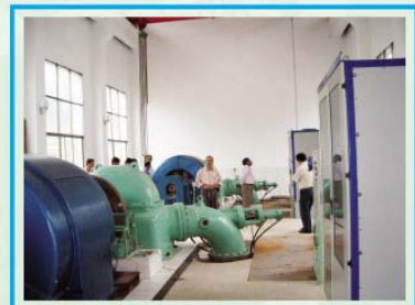
Hunan Sanhekou Powerstation with 3x1MW Inclined-jet Turbine Units
