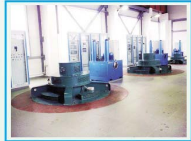
Powerstation with 3 x 2MW Units in Karatal River of Kazakhstan
